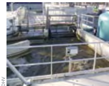
Waste water treatment plant, Varsseveld
